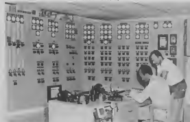
INTERIOR VIEW of Powerhouse No. 1 panel enclosure, with operator's desk and part of panel.
